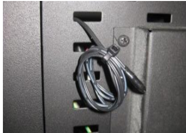
Figure 15 - Room temperature probe
