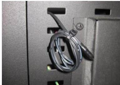
Figure 15 - Room temperature probe
